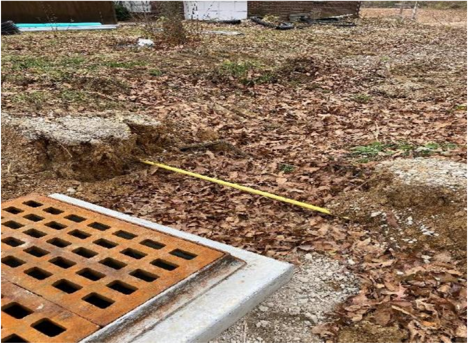
Exposed gas line near Youth House (near new water drain) requiring concrete wrapping
